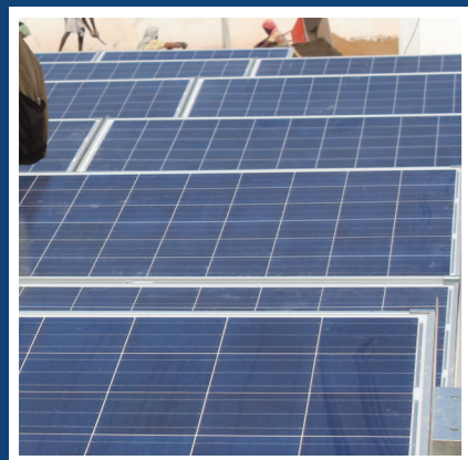
10 KW ON-GRID SYSTEM AT PERUMBAKKAM, CHENNAI
