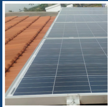
2 KW ON ELEVATED SHED TYPE STRUCTURE AT TRICHY
