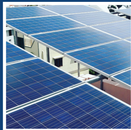
6.5 KW HIGH RISE SOLAR INSTALLATION AT PURASAIWALKAM, CHENNAI
