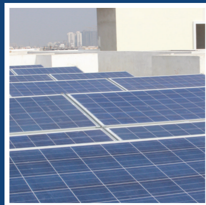
10 KW ON-GRID SYSTEM AT PERUMBAKKAM, CHENNAI
