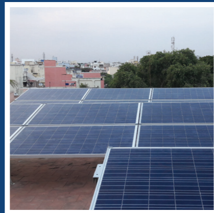
5 KW ON-GRID AT PORUR, CHENNAI
